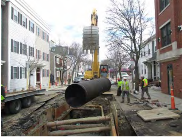
48-inch Storm Drain Installation on E. Third Street Reserved Channel Sewer Separation Contract 3B
