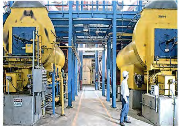
Figure 1: Dryer Furnace Trains
