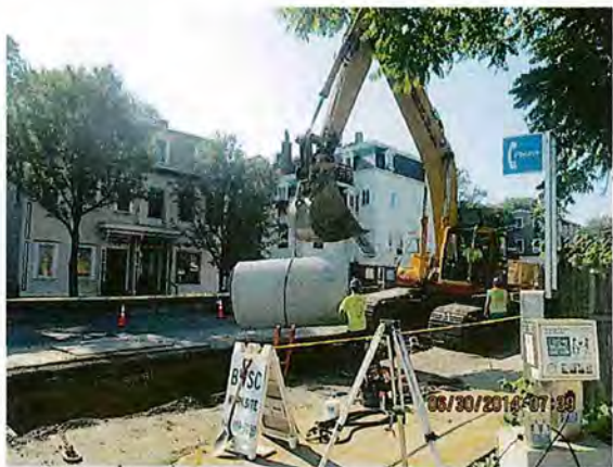
48-inch Storm Drain Installation on L Street Reserved Channel Sewer Separation Contract 4
