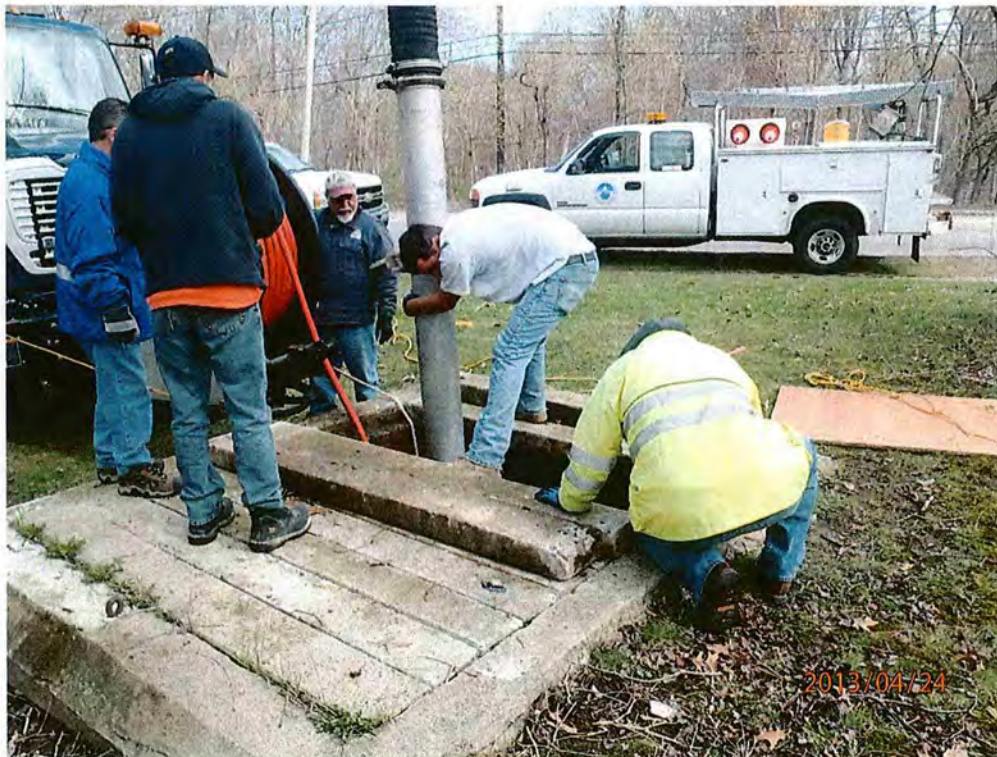
MWRA staff jetting and vacuuming the upstream siphon headhouse structure in MWRA's 30-inch-diameter Section 532 of the Neponset Valley Relief Sewer.
