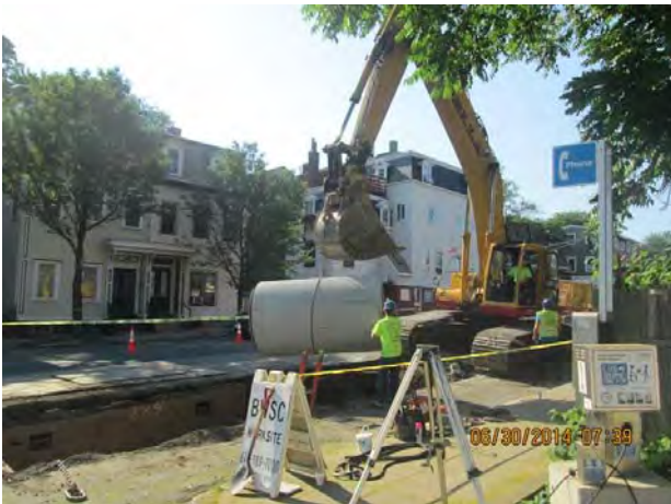
48-inch Storm Drain Installation on L Street Reserved Channel Sewer Separation Contract 4
