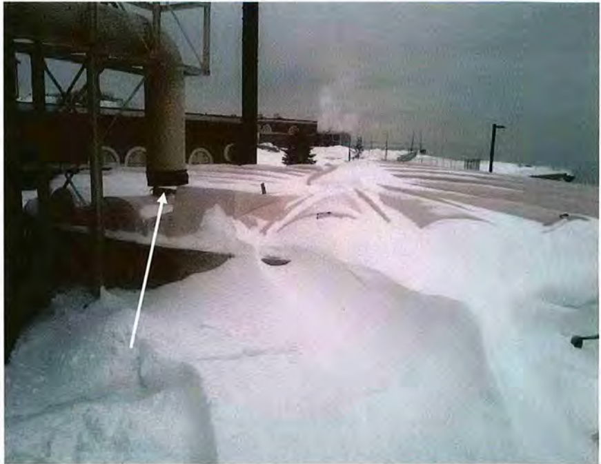
Collapsed Roof On Gravity Thickener; Separation From Air Duct Can Be Seen.
