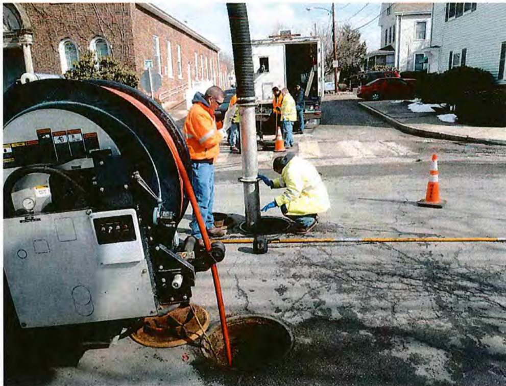
MWRA staff using a Vactor jet to clean and vacuum debris from a blocked City of Waltham 12-inch sewer line in March 2013. Also pictured in background is MWRA's television inspection crew/truck to verify cleaning.
