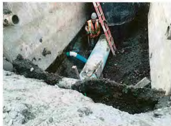
Blakeslee Street Drain Installation Under Water Main CAM004 Sewer Separation Contract 8B
