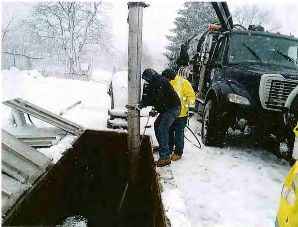
MWRA staff removing grit and sediment from a blocked septage collection tank in Randolph in March 2013. The vactor jet is vacuuming up sediment and grit into the truck's tank.
