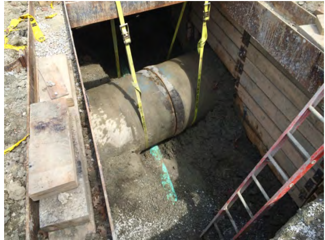
Blakeslee Street Drain Installation Under Water Main CAM004 Sewer Separation Contract 8B
