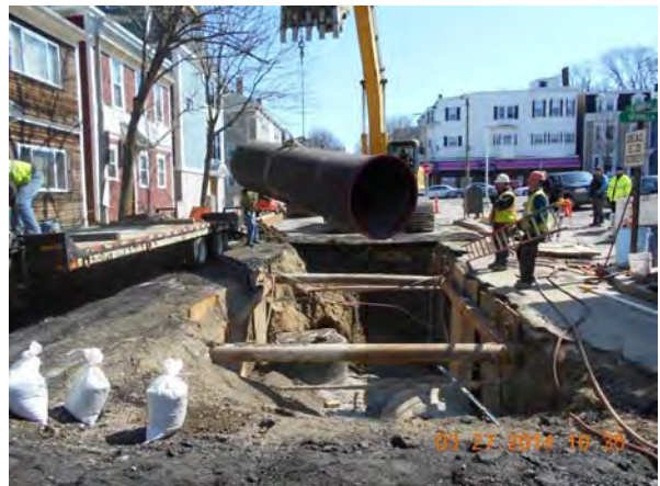
Installation of 48-inch Drain on E. Third Street Reserved Channel Sewer Separation Contract 3B
