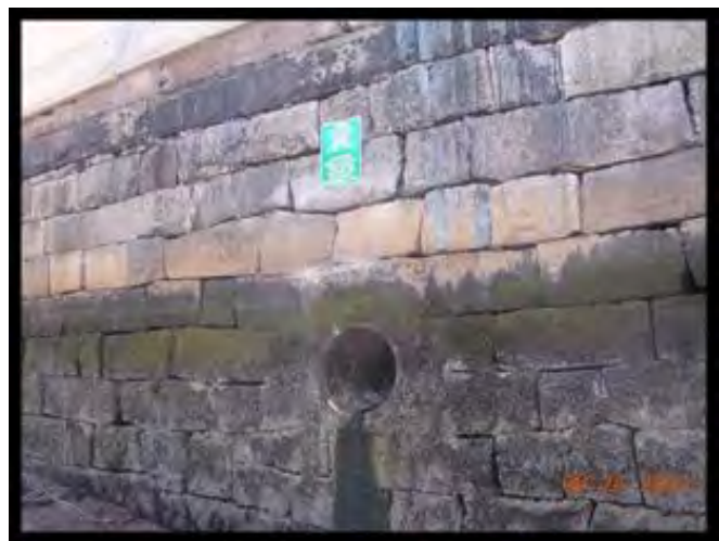
Outfall pipe below high tide water elevation of Mystic River/Chelsea Creek Confluence is now a stormwater outlet.
