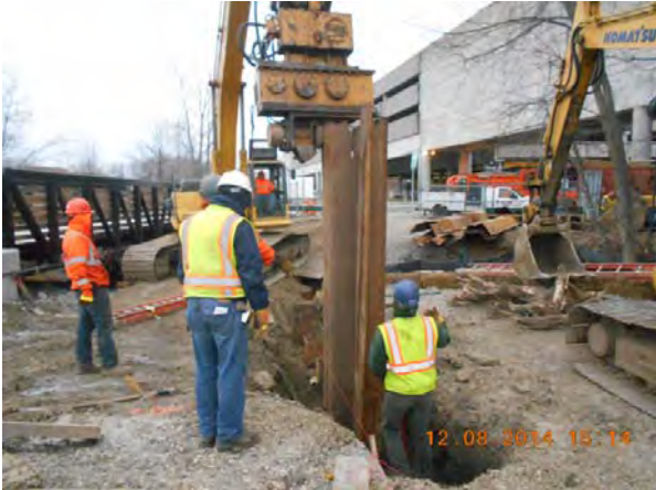
Installation of Steel Sheet Piling for Excavation Support 48-inch Rindge Ave. Siphon at Outfall MWR003
