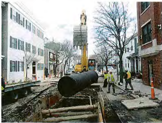
48-inch Storm Drain Installation on E. Third Street Reserved Channel Sewer Separation Contract 3B
