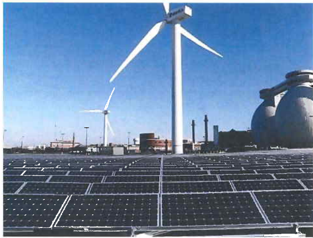
DITP Parking Lot PV
