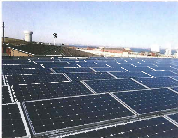
DITP Grit Roof PV
