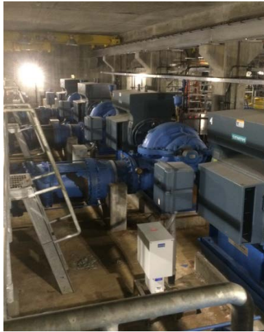
Chestnut Hill Emergency Pump Station
