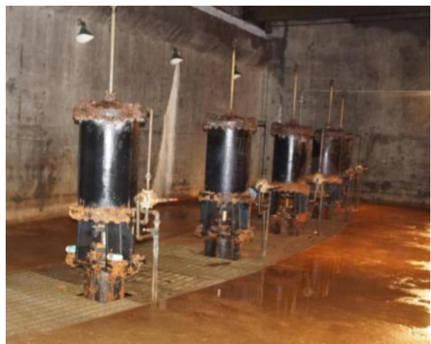
Shaft 7 valve actuators
