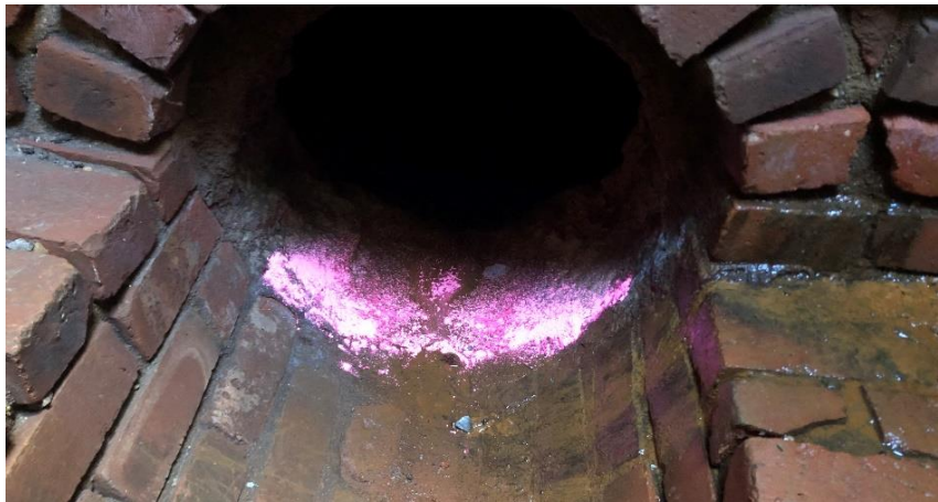
Figure 8-3. Chalking Applied to the Overflow Pipe at RE070/8-8
