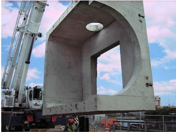
Placement of tidegate chamber at Outfall 076 on Papas Way
