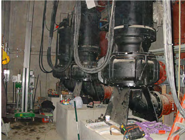
Three 250 hp pumps that are located in the pump room of the dewatering pump station at Massport's Conley Terminal
