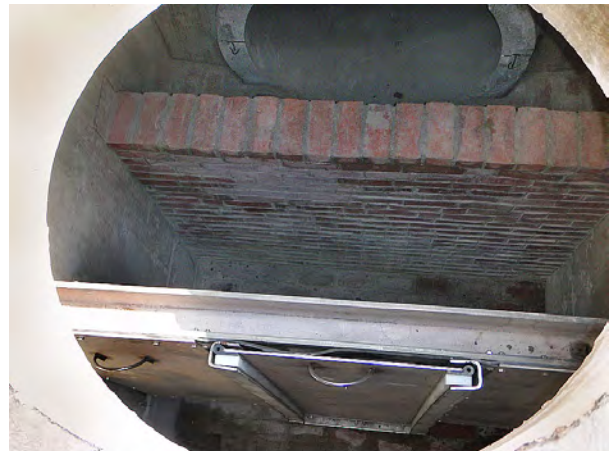
New underflow baffle for floatables control at RE-003-2 in Maverick & Cottage, East Boston
