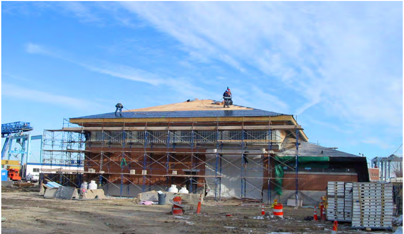
15 mgd dewatering pump station for the North Dorchester Bay CSO storage tunnel at Massport's Conley Terminal
