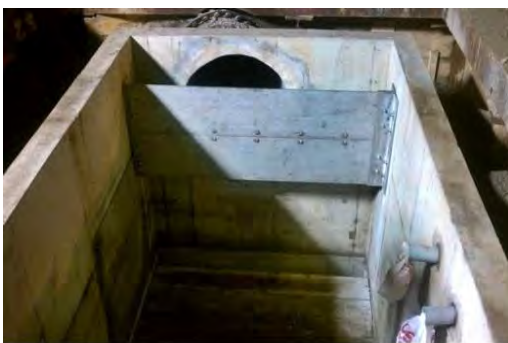
CAM 002A & B inlet structure-baffle is visible in front of CAM 002A outlet with a steel plate (temporary condition) bolted on the left hand wall on the CAM 002B outlet.
