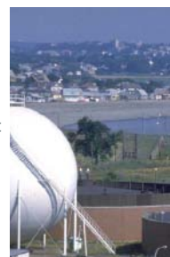
Primary wastewater treatment plant built on Deer Island to handle the metropolitan Boston sewage
