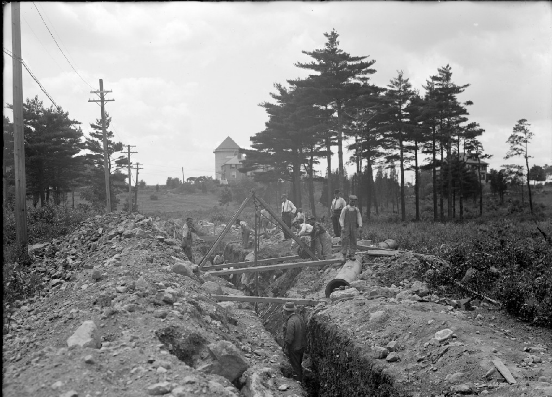
M. EX. H. S. P. L. SEC. 36, LAYING 16" MAIN, ROBBINS RD. NEAR HAWTHORNE AVE. ARLINGTON. JUNE 25, 1910. 6563
