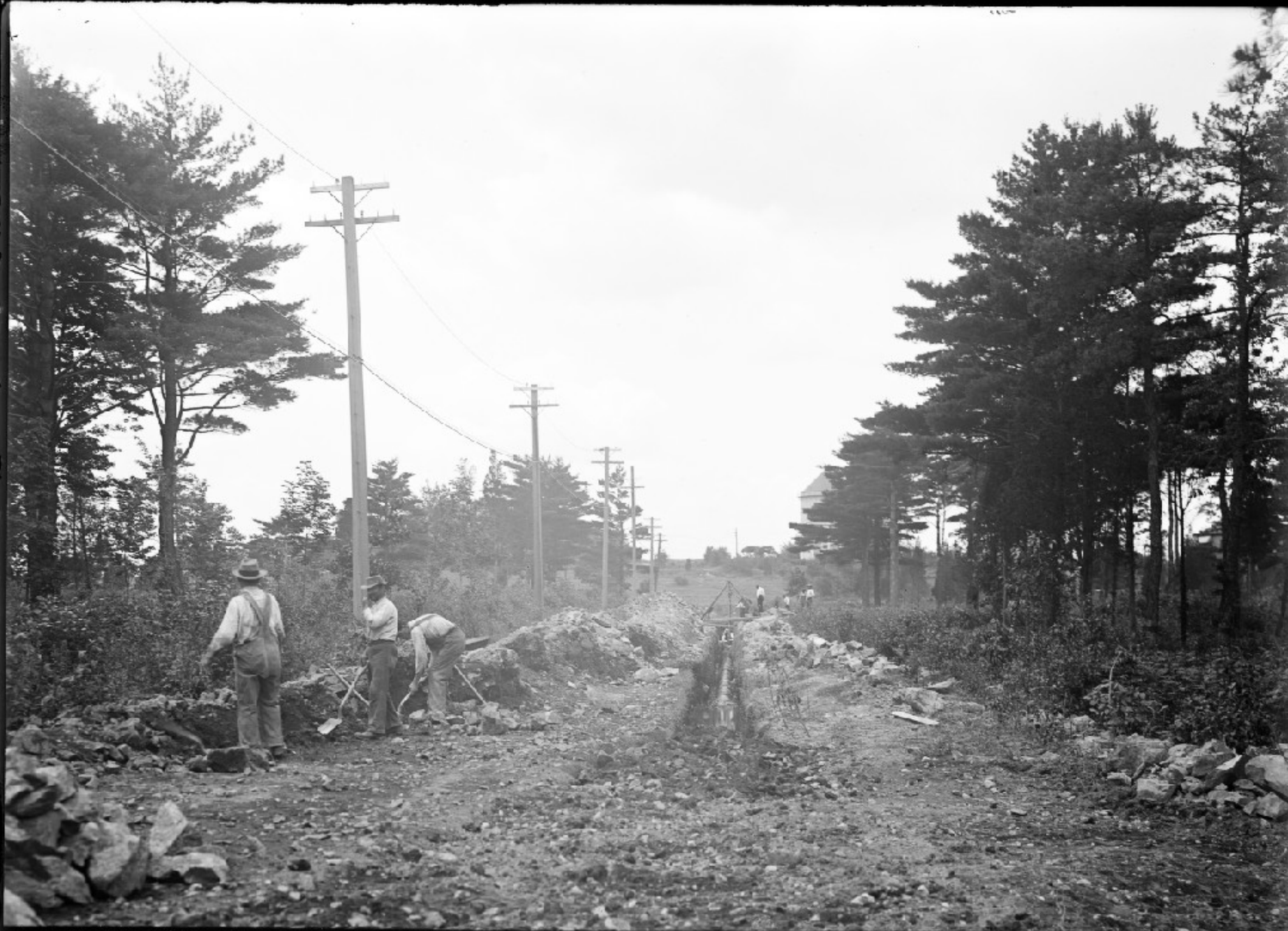
N. EX. H. S. P. L. SEC. 36, REFILLING 16" PIPE TRENCH, ROBBINS RD. NEAR HAWTHORNE 6564 AVE. ARLINGTON. JUNE 25, 1910.
