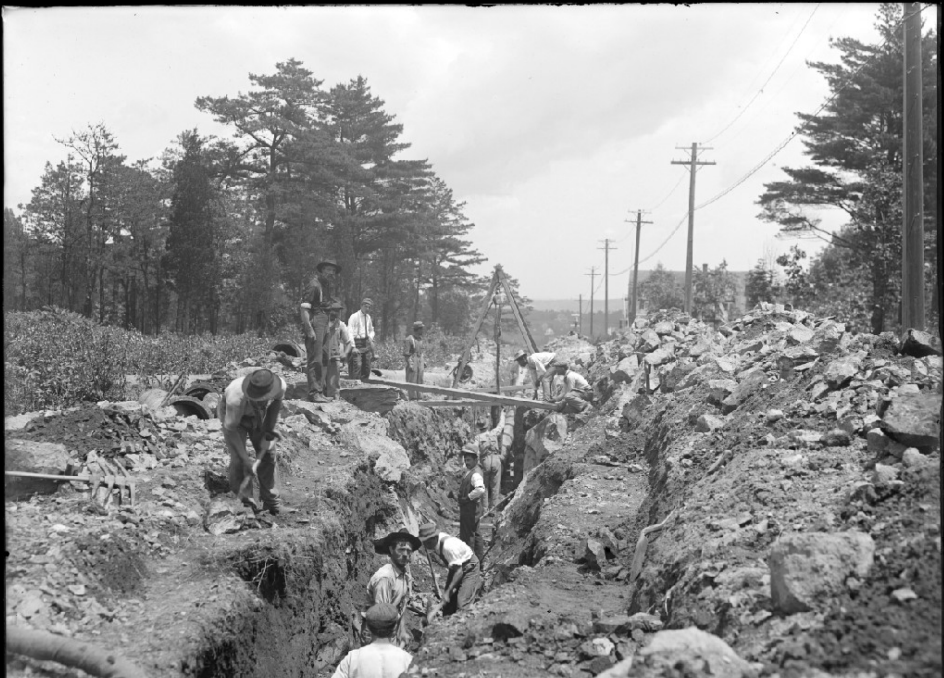
W. EX. H. S. P. L. SEC. 36, LAYING 16" MAIN IN ROCK TRENCH, ROBBINS RD. ARLINGTON. JUNE 25, 1910. 6582
