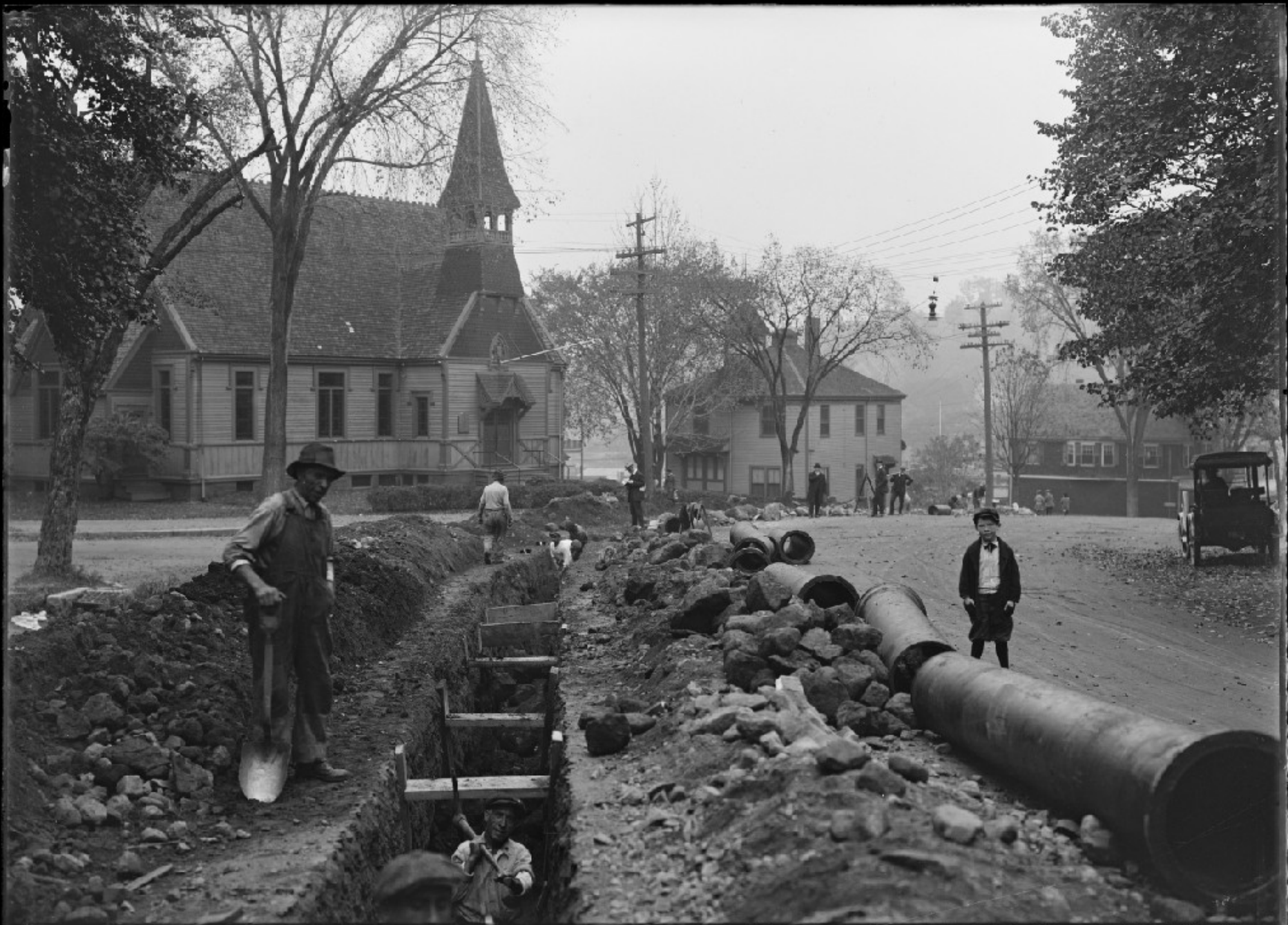
N. EX. H. S. P. L. SEC. 45 ARLINGTON. 16 IN. PIPE TRENCH COR. OF PARK AV. & PAUL REVERE RD. OCT. 16, 1919. 7604
