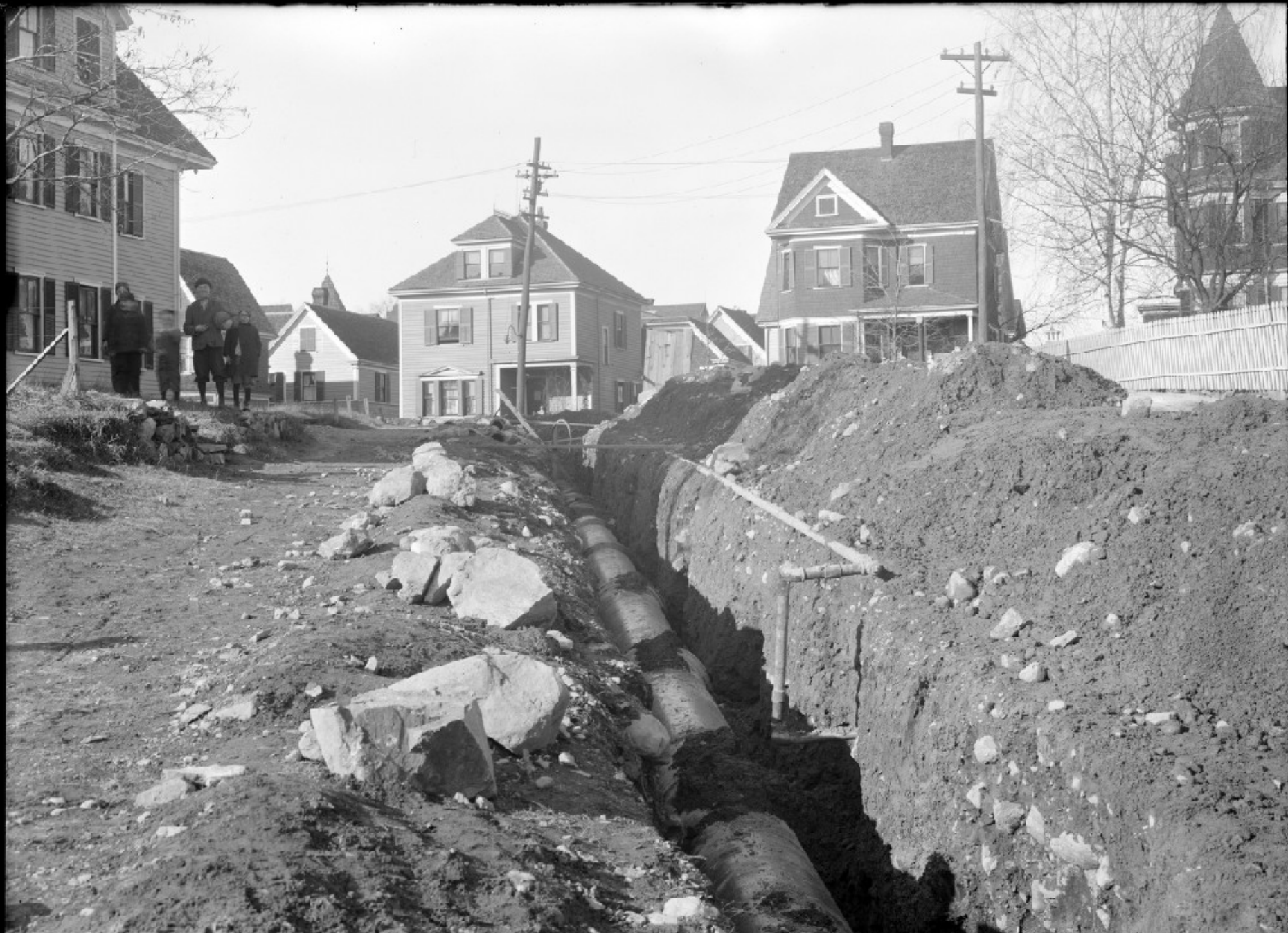
N. H. S. PIPE LINES SEC. 33. ARLINGTON ST. NEAR FOSTER STREET, EVERETT. 24" WATER PIPE IN TRENCH. NOV. 27, 1909. 6443
