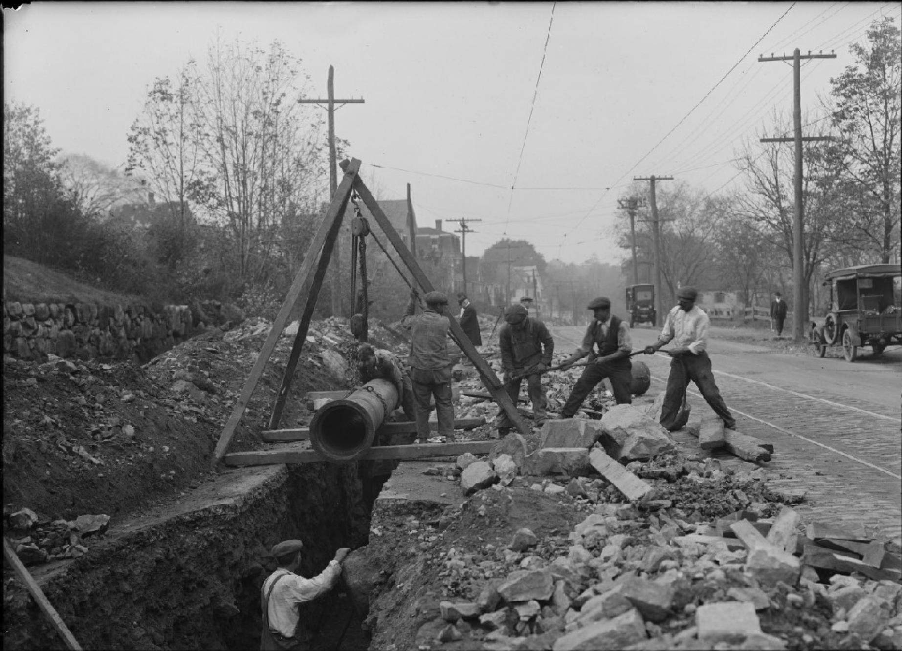
N. EX. H. S. P. L. SEC. 45 ARLINGTON. LAYING 16 IN. PIPE MASS AV, NEAR DUNDIE RD. OCT, 16, 1919. 7605
