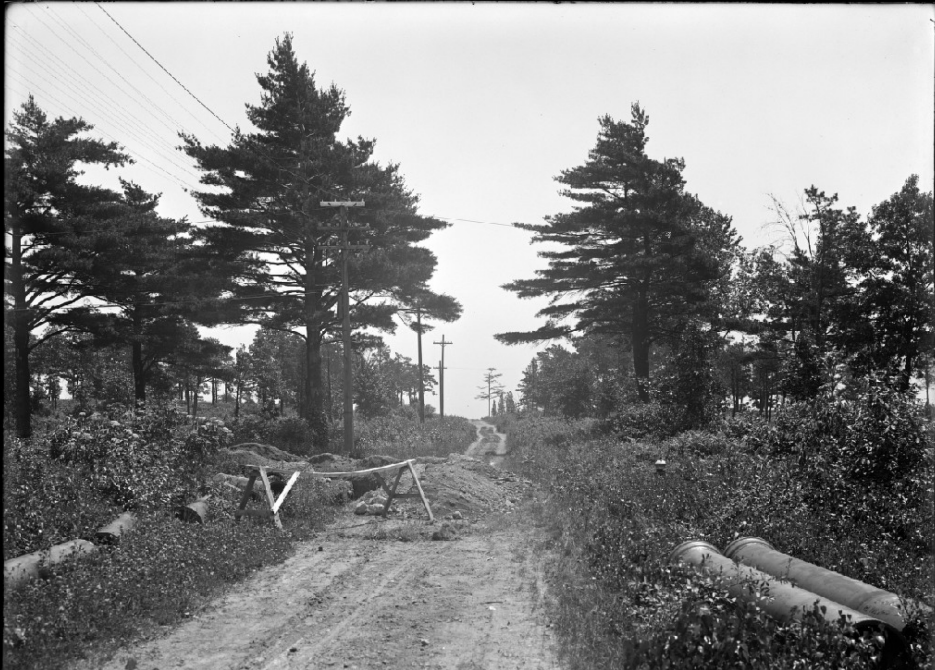
N. EX. H. S. P. L. SEC. 36, TRENCH FOR 16" MAIN COR. HAWTHORNE AVE. & ROBBINS RD. 8560 ARLINGTON. JUNE 26, 1910.
