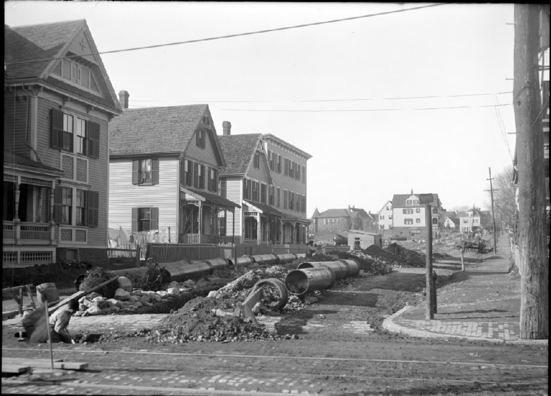
N. H. S. PIPE LINES SEC. 33, ARLINGTON ST. FROM FERRY ST. EVERETT. CONDITION OF STREET NOV. 27, 1909. DURING CONSTRUCTION OF 24" WATER MAIN. 6442
