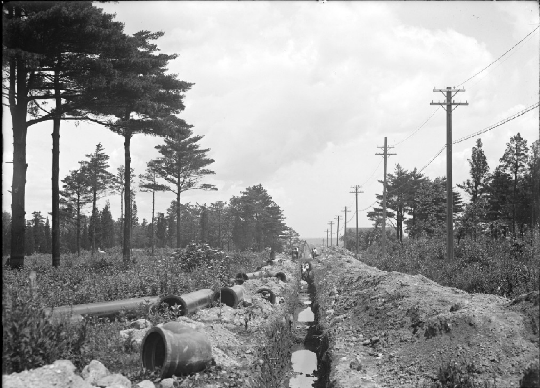
N. EX. H. S. P. L. SEC. 36, LAYING 16" MAIN, ROBBINS RD. NEAR HAWTHORNE AVE. ARLINGTON. JUNE 25, 1910. 6561
