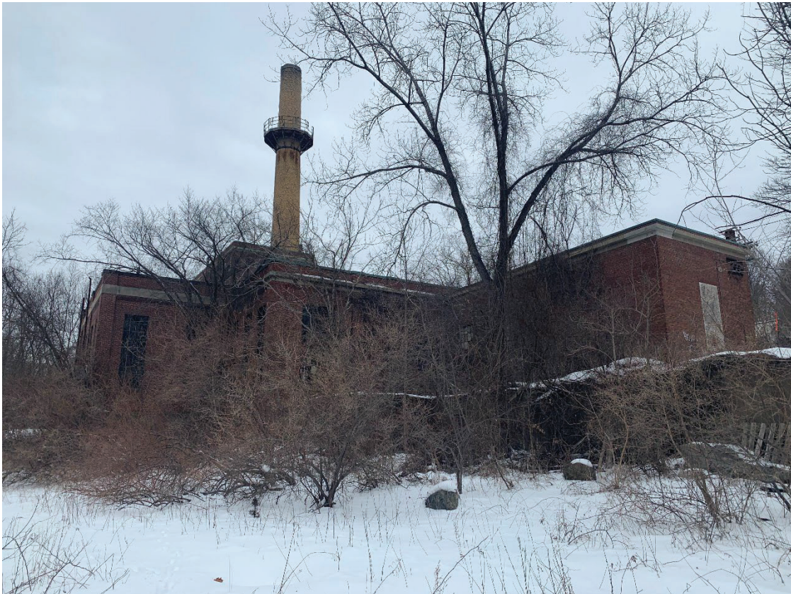
13. Lower Fernald Property Site – east and south elevations of power plant (WLT.935)
