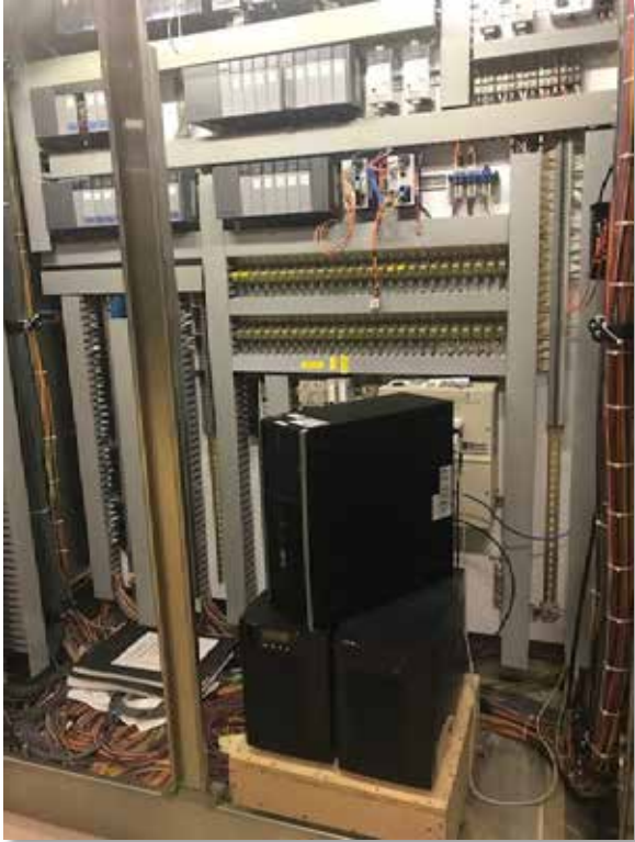
An Existing panel and UPS
