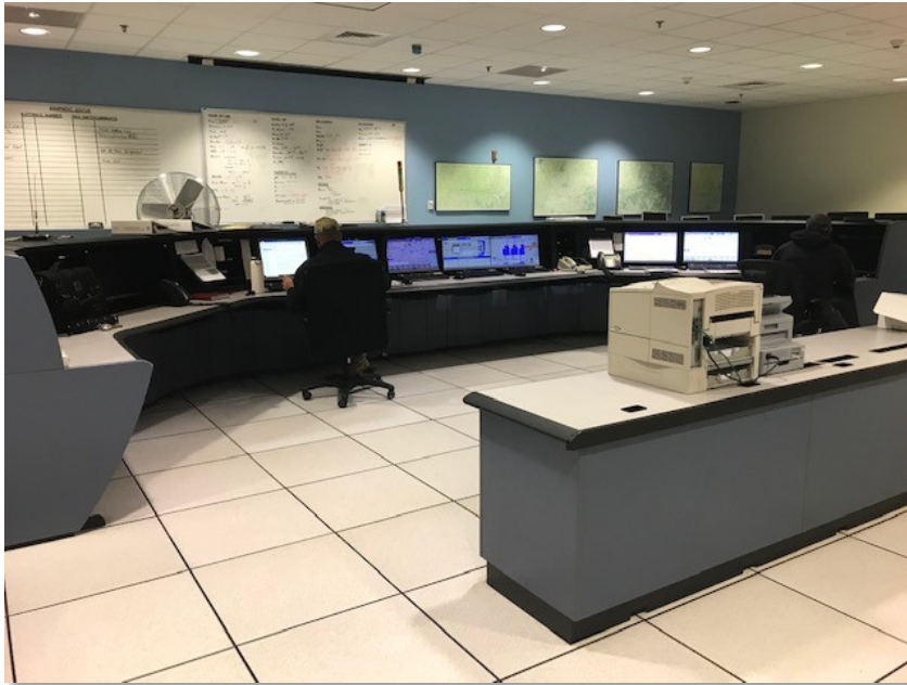
Existing Control Room
