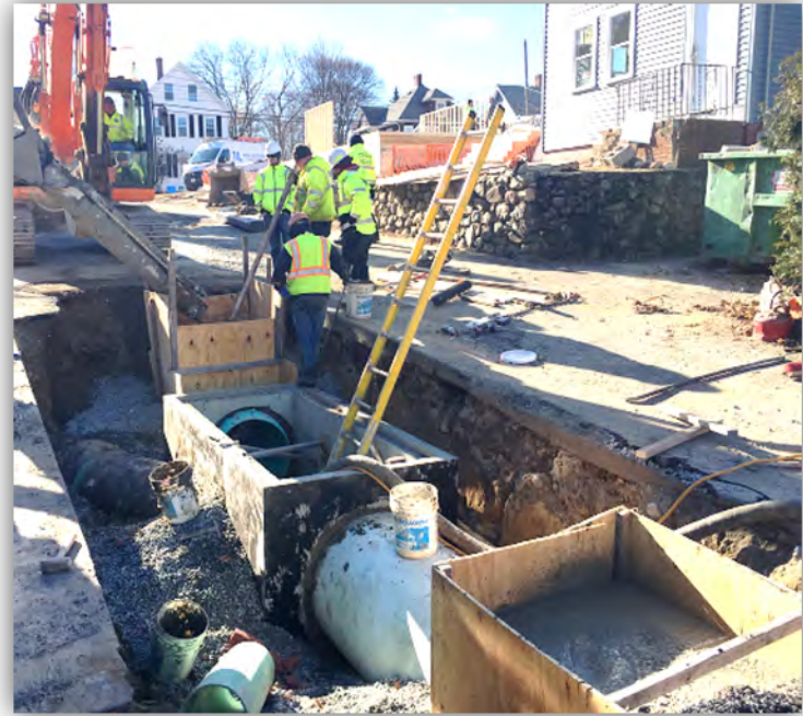
New 30-inch PVC drain line
