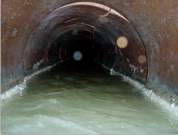
Sewer Rehabilitation Needed to Address Pipeline Defects
