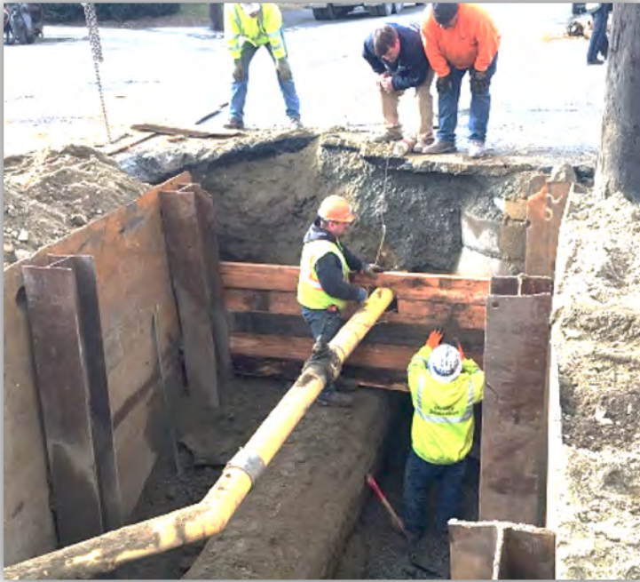
Gas main installed directly over culvert
