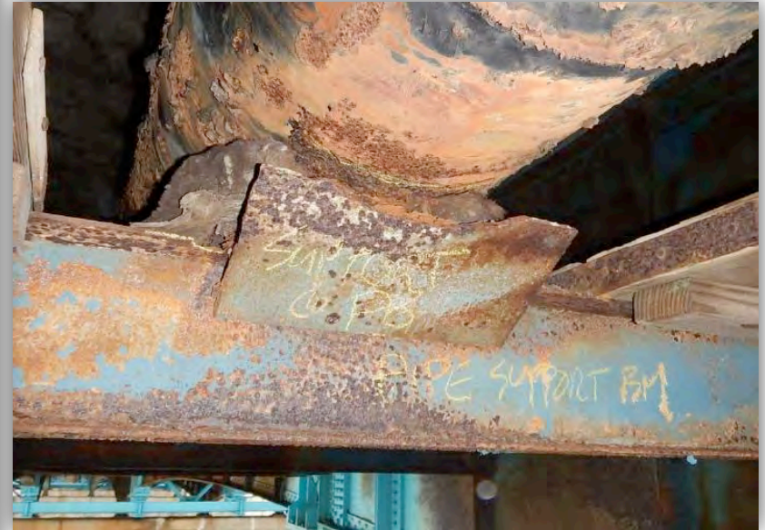
Deteriorated Pipe Support and Beams
