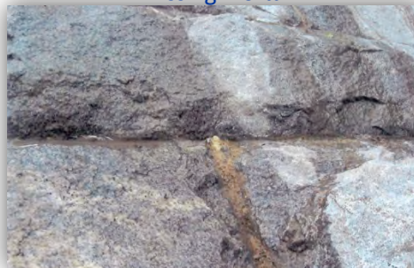
Clogged weep hole
