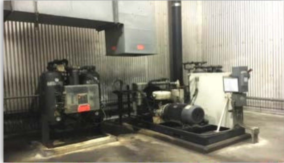
Air Compressor System
