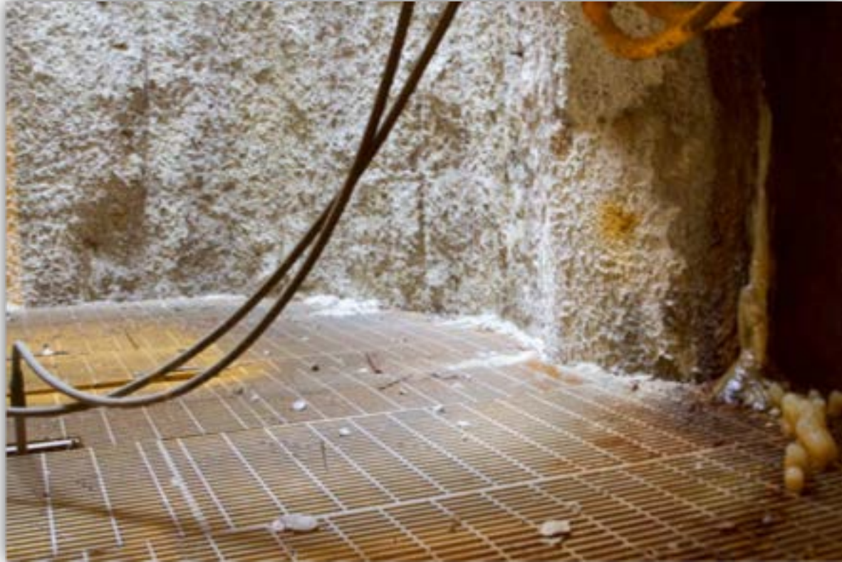
Deteriorated Concrete in Shaft at Chelsea Creek Headworks
