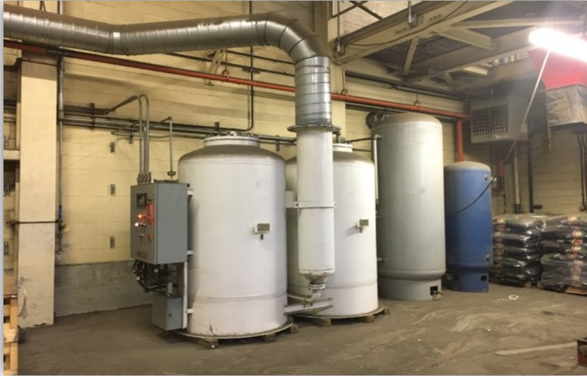
Nitrogen Purge Generator (fire suppression system)
