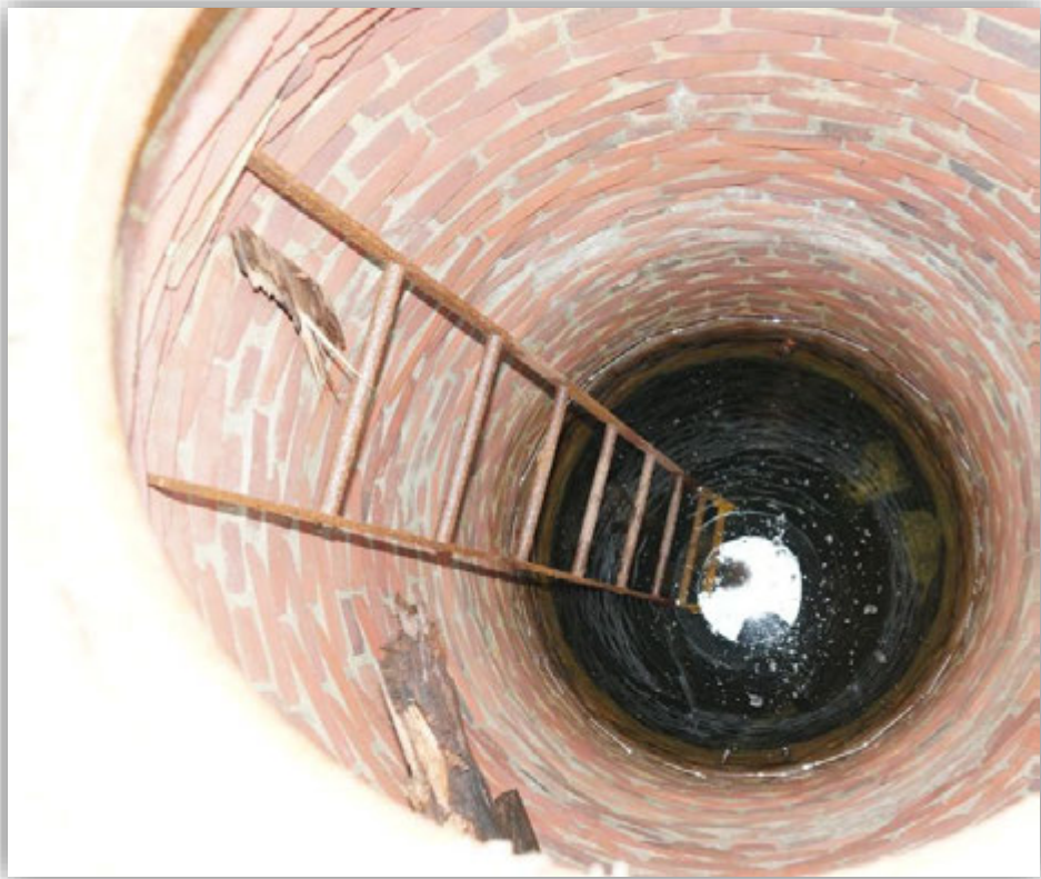
Shaft 7D connecting pipe air valve chamber
