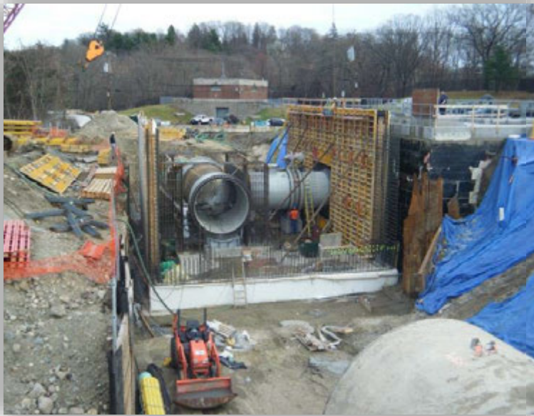
New valve chamber connecting MWWST and Hultman Aqueduct at Shaft 5 (2013)
