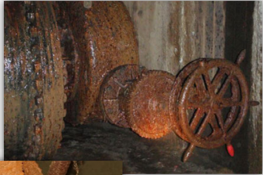
Cone Valve at Shaft 7B
