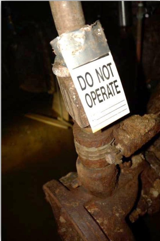
Shaft 8 PRV Chamber
