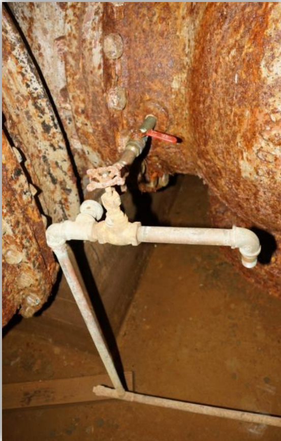
Control piping at Shaft 8
