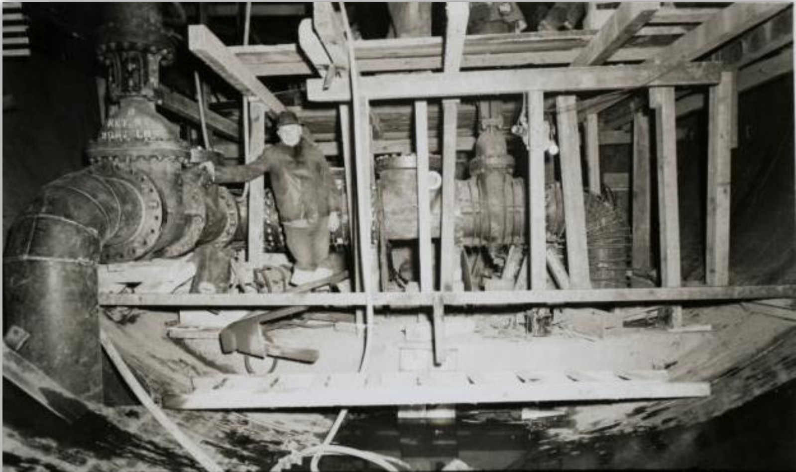
16" hydraulic valves and fittings - Looking N'ly from shaft - Shaft #9 - City Tunnel Ext. - Contract 193 - 2/3/58 - 193-181 Photo Barbier -
