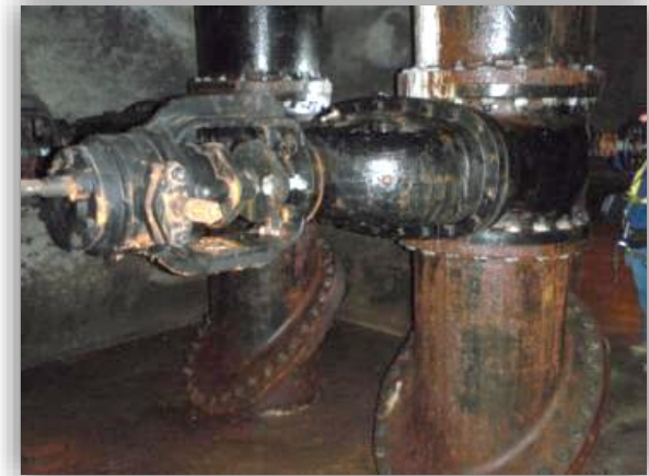
20-inch Shaft 7 Valve
