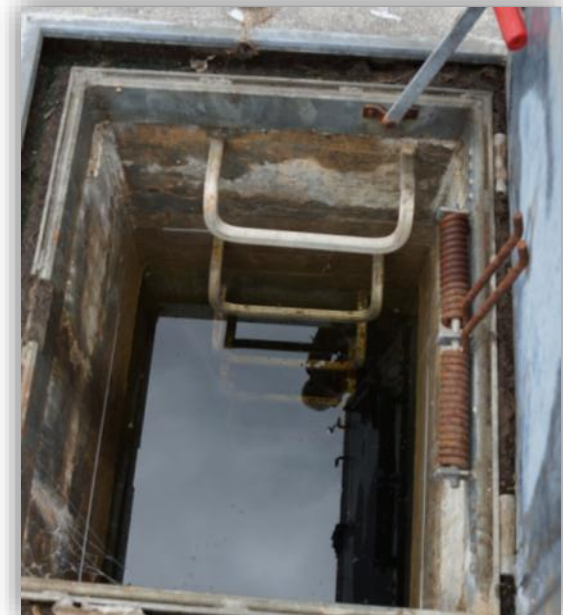
Chamber at Shaft 7D
