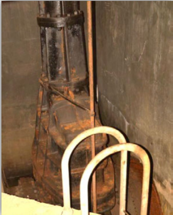
60-inch gate valve Shaft 5
