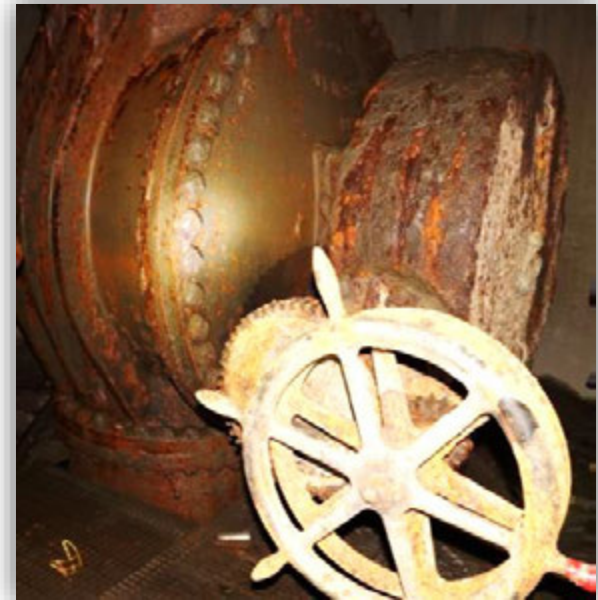
Cone Valve at Shaft 7B
