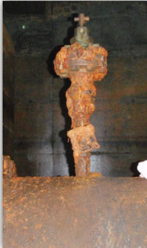
Air valve at Shaft 9A
