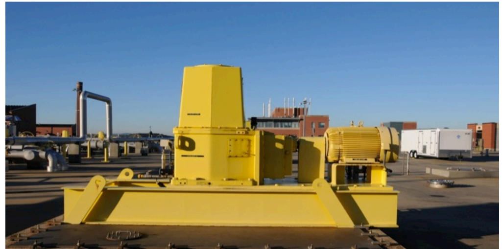
Typical Reactor Mixer Motor/Gearbox
