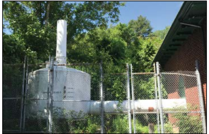
Figure 4: Odor Control Adsorber System
