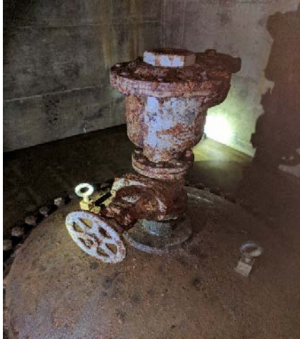
Shaft Cap and Air Valve at Shaft 8
