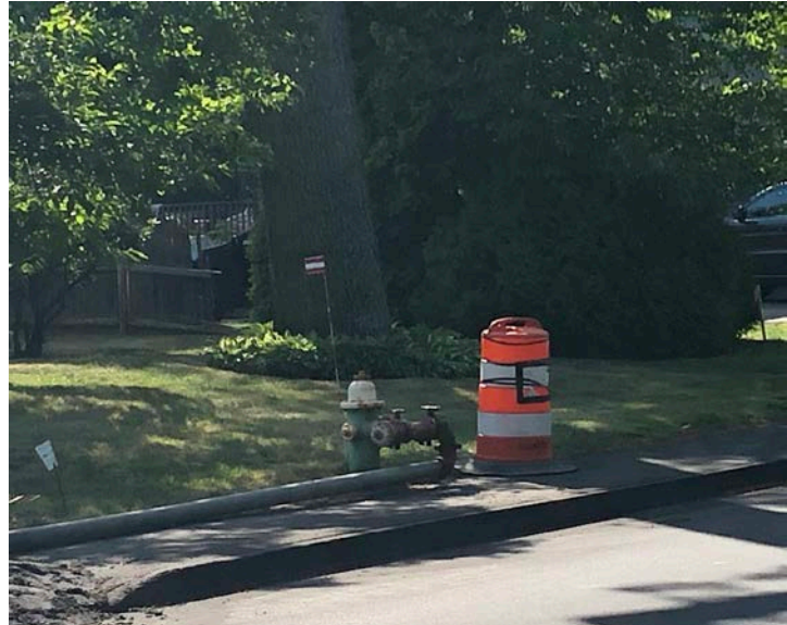
Figure 1: LCWD Hydrant Connection
