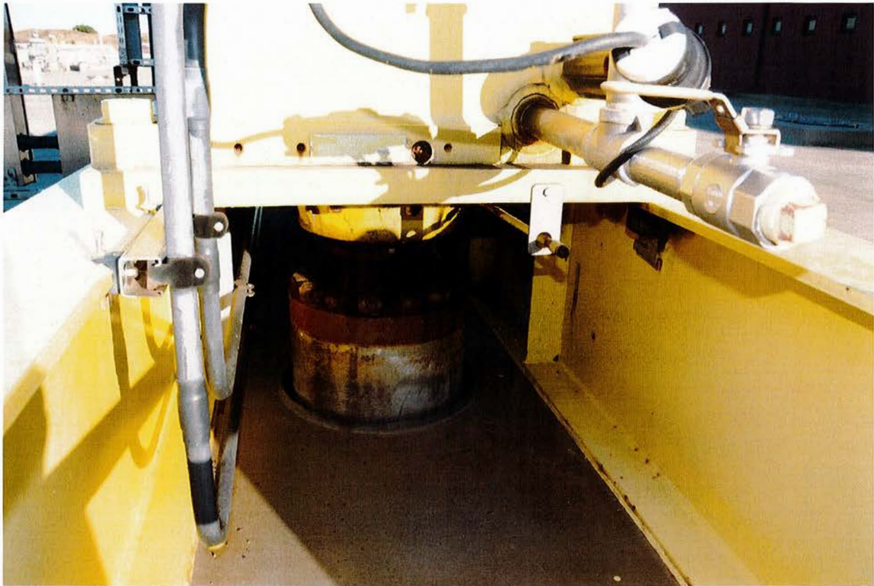
Picture depicts the top of one of the aerator/mixer shafts where it connects with the triple-reduction gearbox
