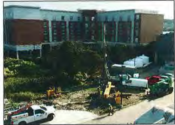
Drilling micropile and preparing for pile load test to confirm pile capacity
