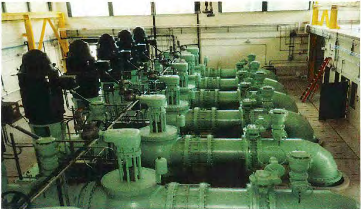
Pump Surge Control Valves
