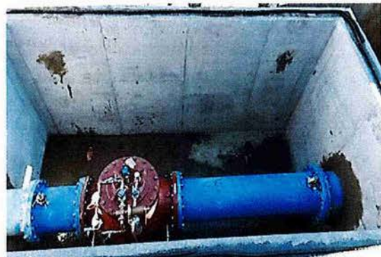
Town of Reading New Control Valve vault downstream of meter
