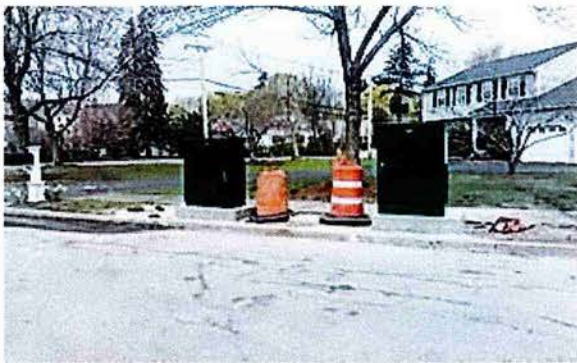
Above ground meter cabinets on Louanis Drive
