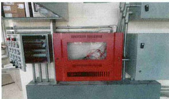
New EST 3 Fire Alarm Panel in the Guard House
