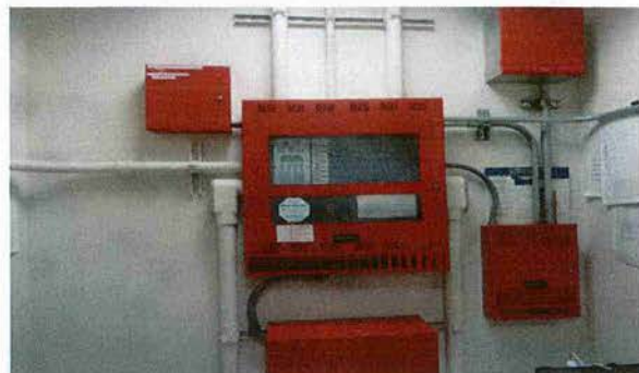
Existing Main EST2 Fire Alarm Panel at Admin. Bldg.
