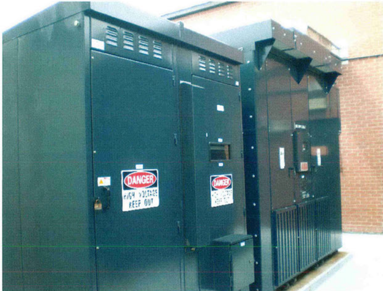
Figure 1-Typical Electrical Substation Equipment
