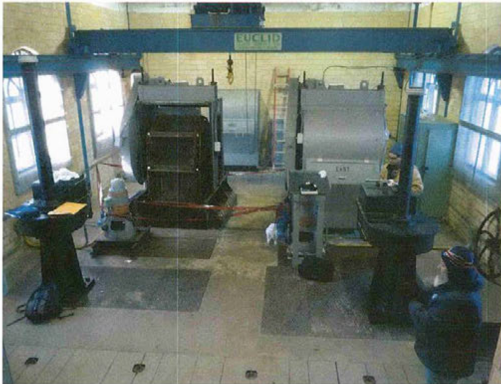
Chicopee Valley Aqueduct Traveling Screens
