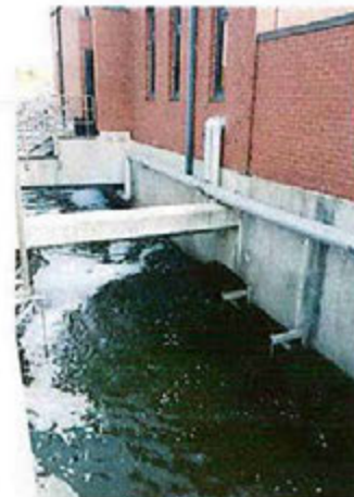
Broken pipe under water during normal flow conditions
