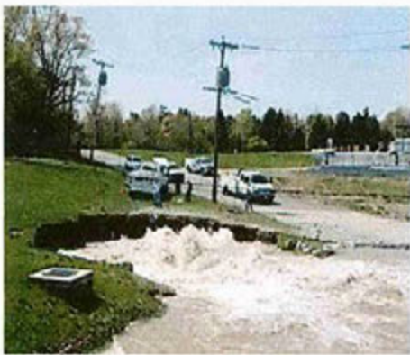
Figure 5: Last used to supplement peak hour demand during Shaft 5A emergency in 2010
