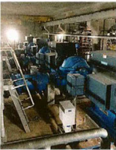
Figure 3: Four 1,000 HP electric pumps in an underground chamber.
