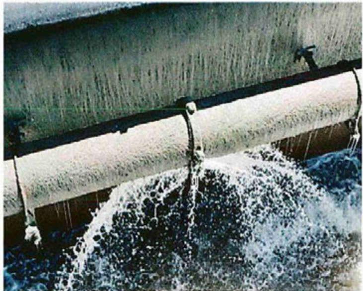
Leaking coupling with channel drained
