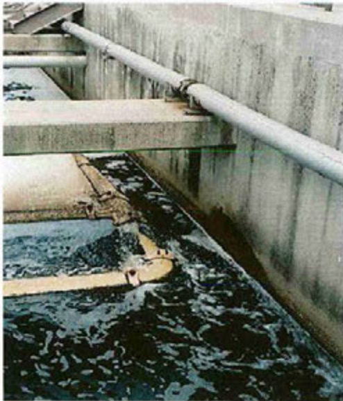
Coupling leaking in channel
