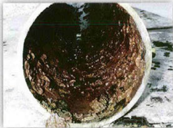
Tuberculated Cast Iron Pipe
