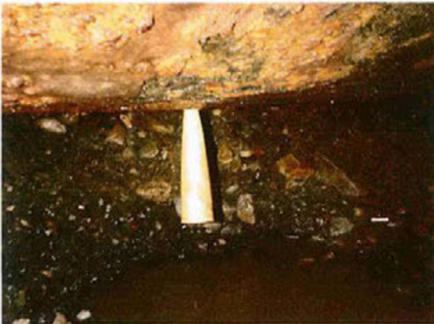
Plugged Leak Prior to Cap Weld
