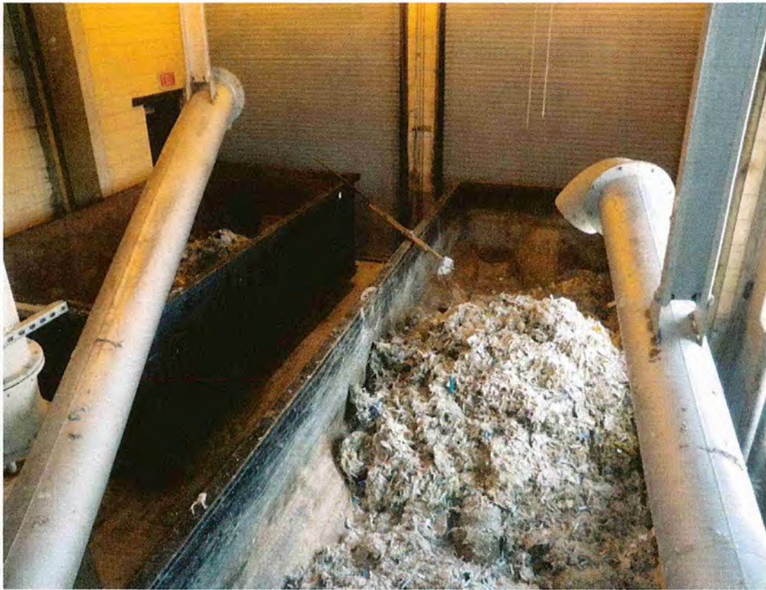
Partially Filled Roll-Off Containers Receiving Washed Screenings from the Removal System Conveyor (Not Shown) Discharge Piping at the Winthrop Terminal Facility
