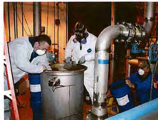
Replacing the Catalyst on an Ozone Destruct Unit at the Carroll Water Treatment Plant
