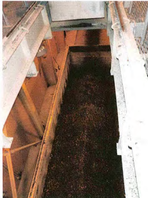
View of Grit Trailer from above Conveyor Drop Opening. Trailer Contains Approximately One Week's Accumulation
