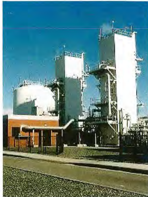
Cryogenic Oxygen Facility at the Deer Island Treatment Plant
