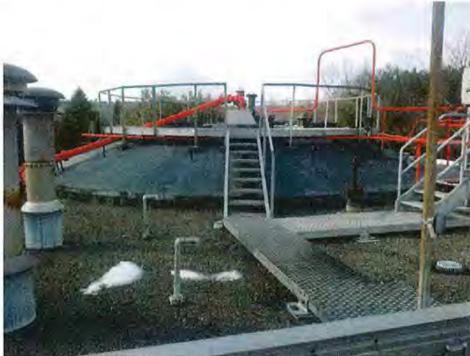
Fixed Cover of One of Two Digesters at the Clinton Advanced Wastewater Treatment Plant
