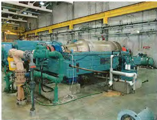
Rotating Assembly Inside an Uncovered Centrifuge
