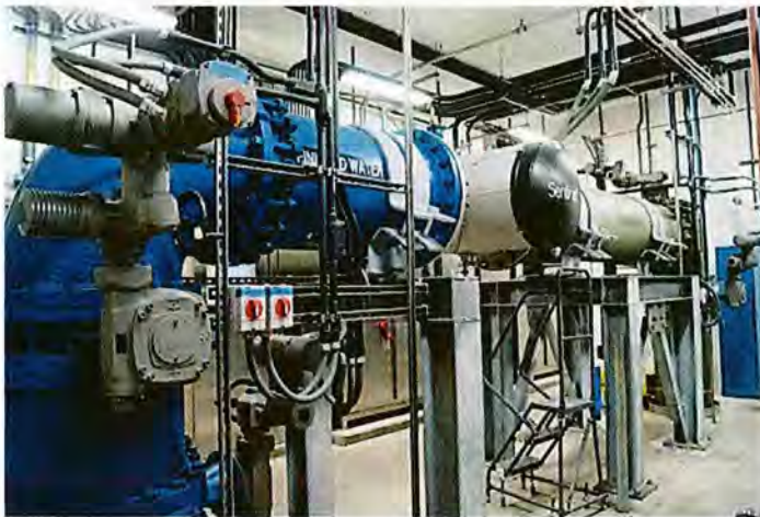
UV Reactors at the William A. Brutsch Water Disinfection Facility
