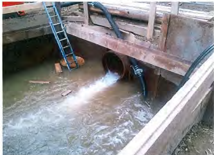
Figure 2. Water leaking into trench.
