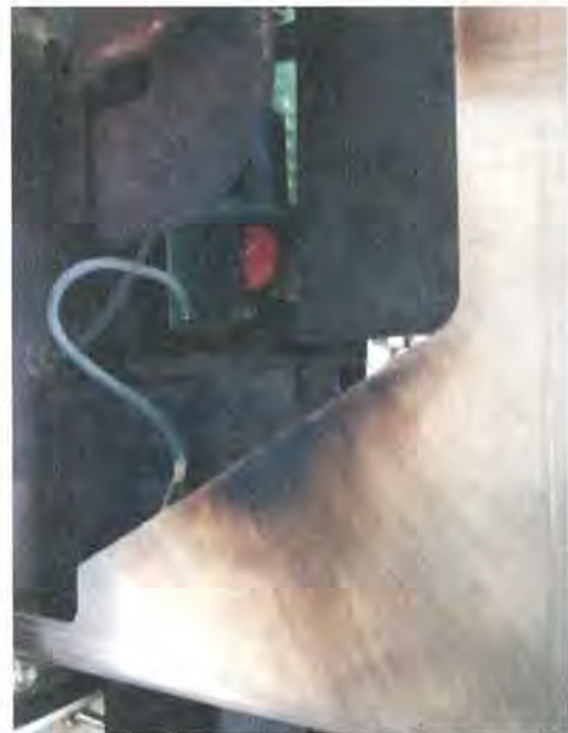
Figure 4: Damage to VFD on Centrifuge 7
