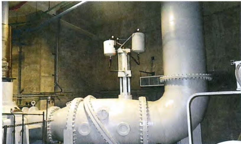
Top-Mounted Dashpot on Check Valve in SSPS
