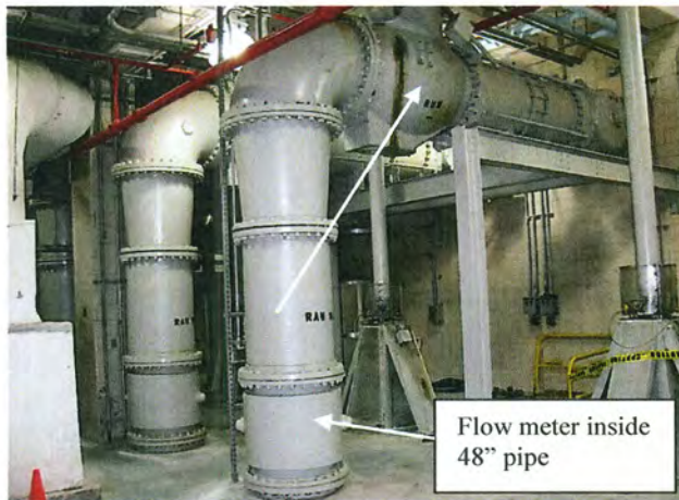
Check Valve and Flow Meter in WTF
