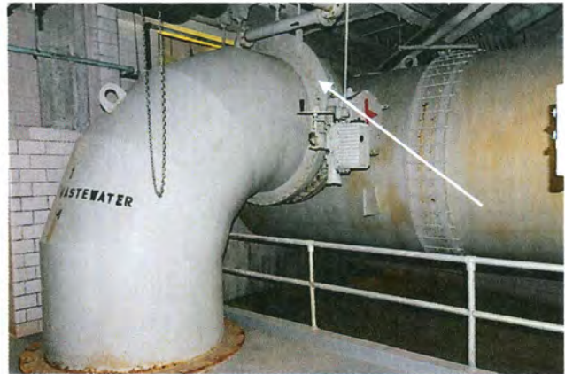
Upper 60-inch Butterfly Valve in NMPS
