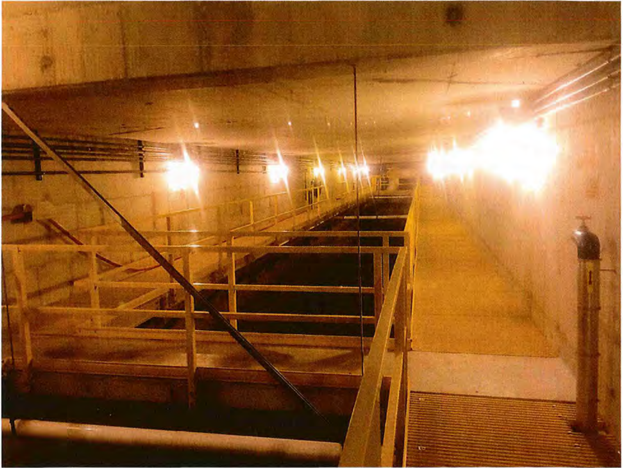
One of Six Channels at the Facility
