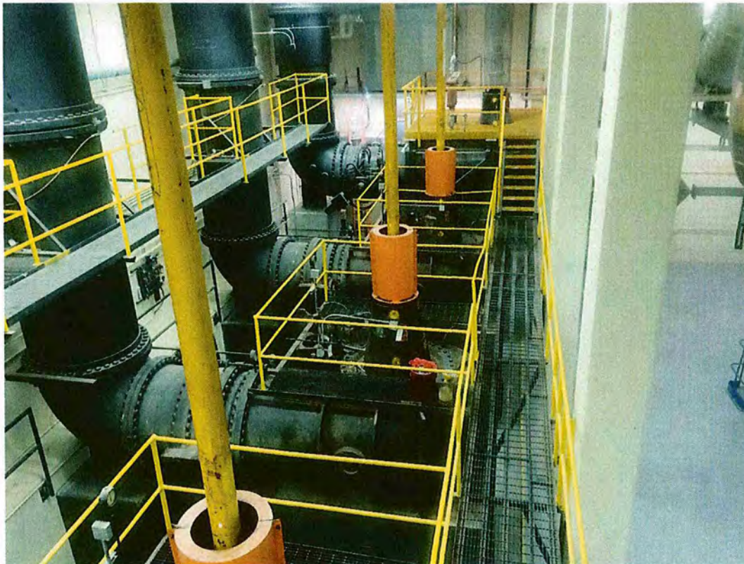
Lower Level: Three Pumps, Shafts, and Discharge Piping
