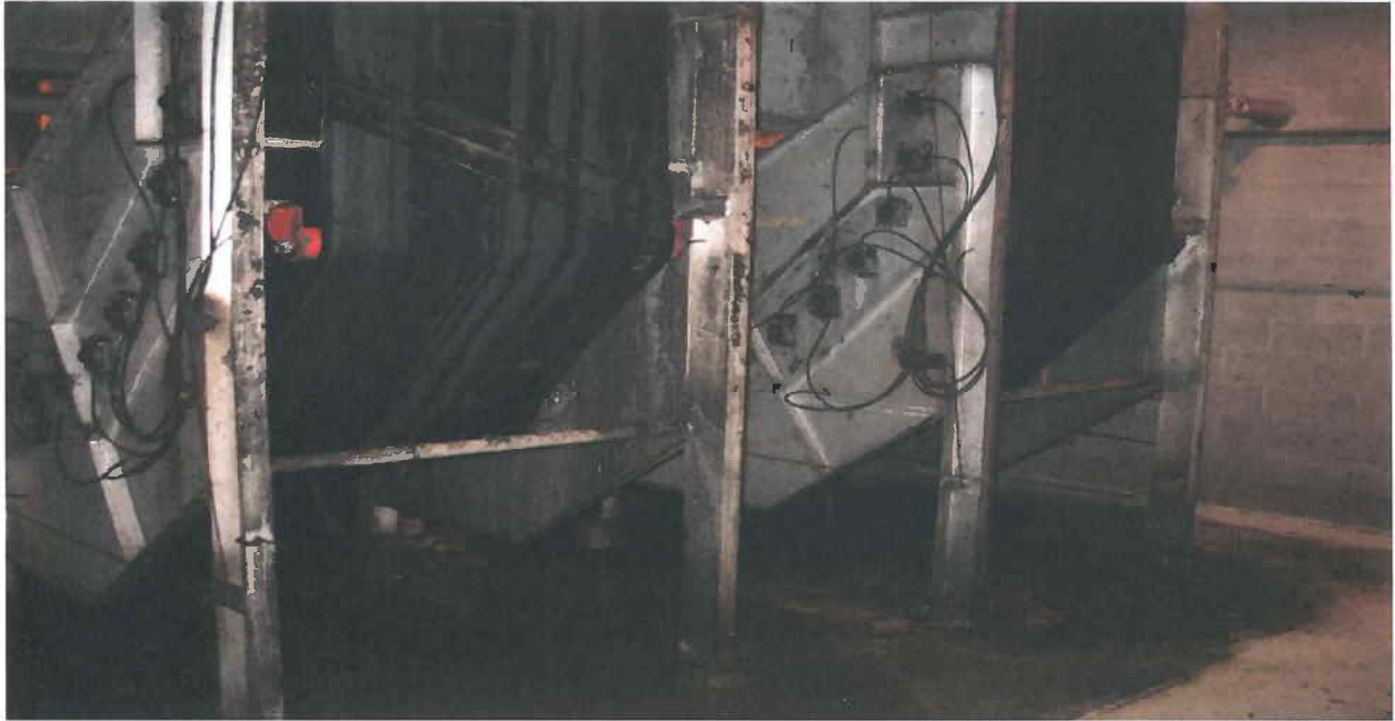
Vertical Screenings Conveyors
