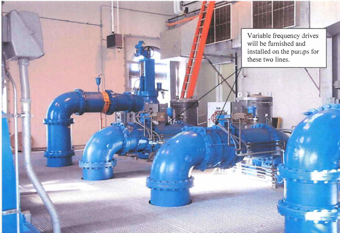
Discharge piping for pumps 4 through 7, left to right (VFDs will be added to Pumps 5 and 6)
