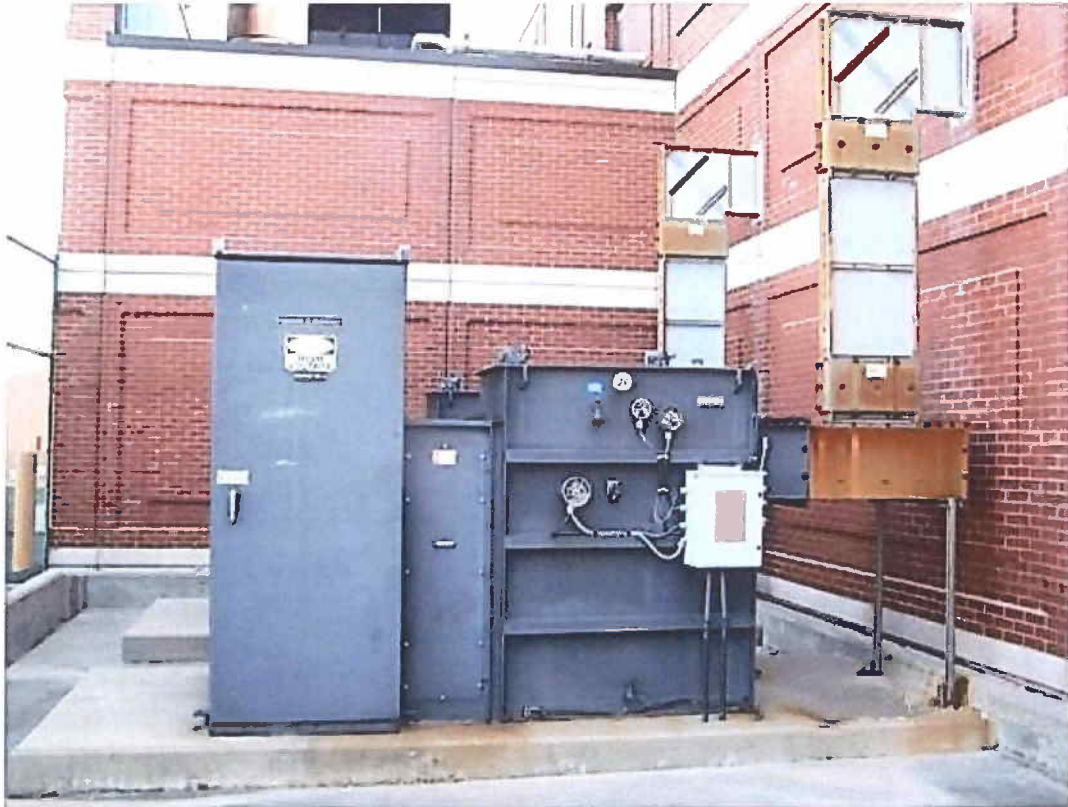
Unit Substation 14D – Load Break Switch, Transformer and Bus Ducts
