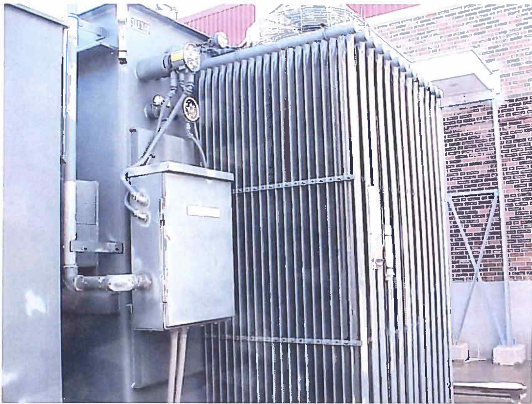
Unit Substation 14A Transformer
