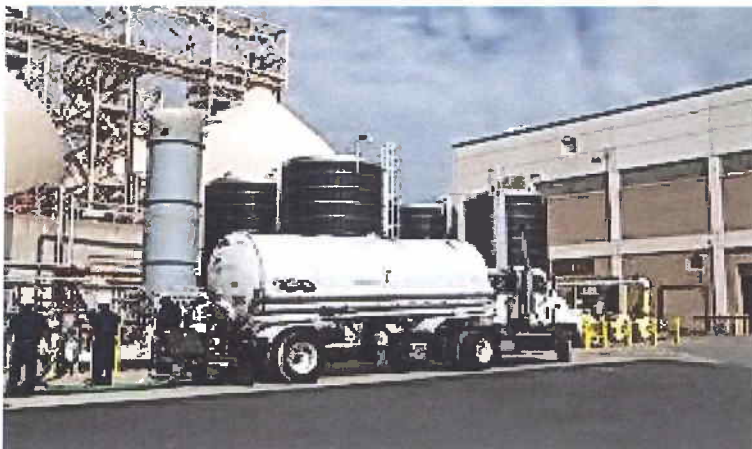
Figure 8: Typical Food Waste Truck Off-Loading Station
