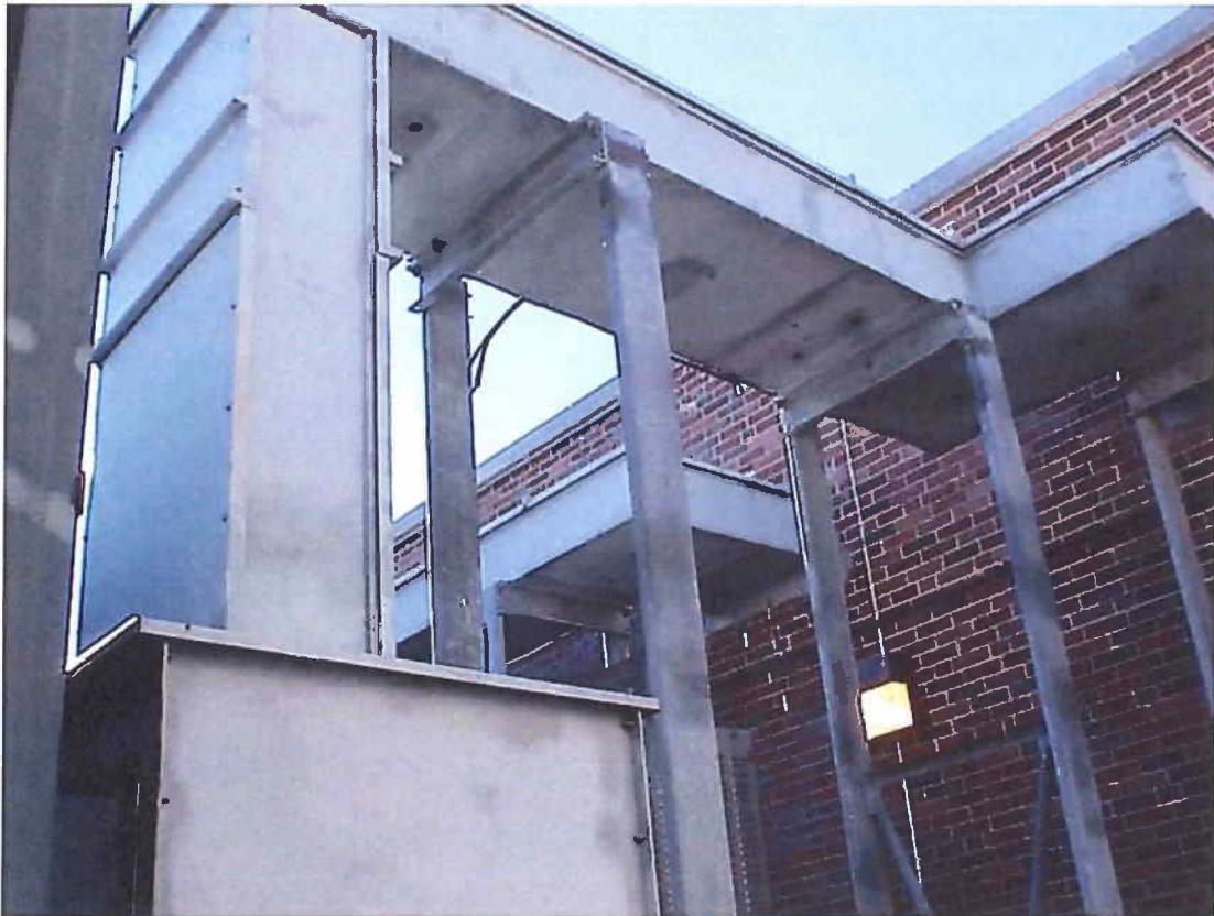
Unit Substation 7 Bus Ducts
