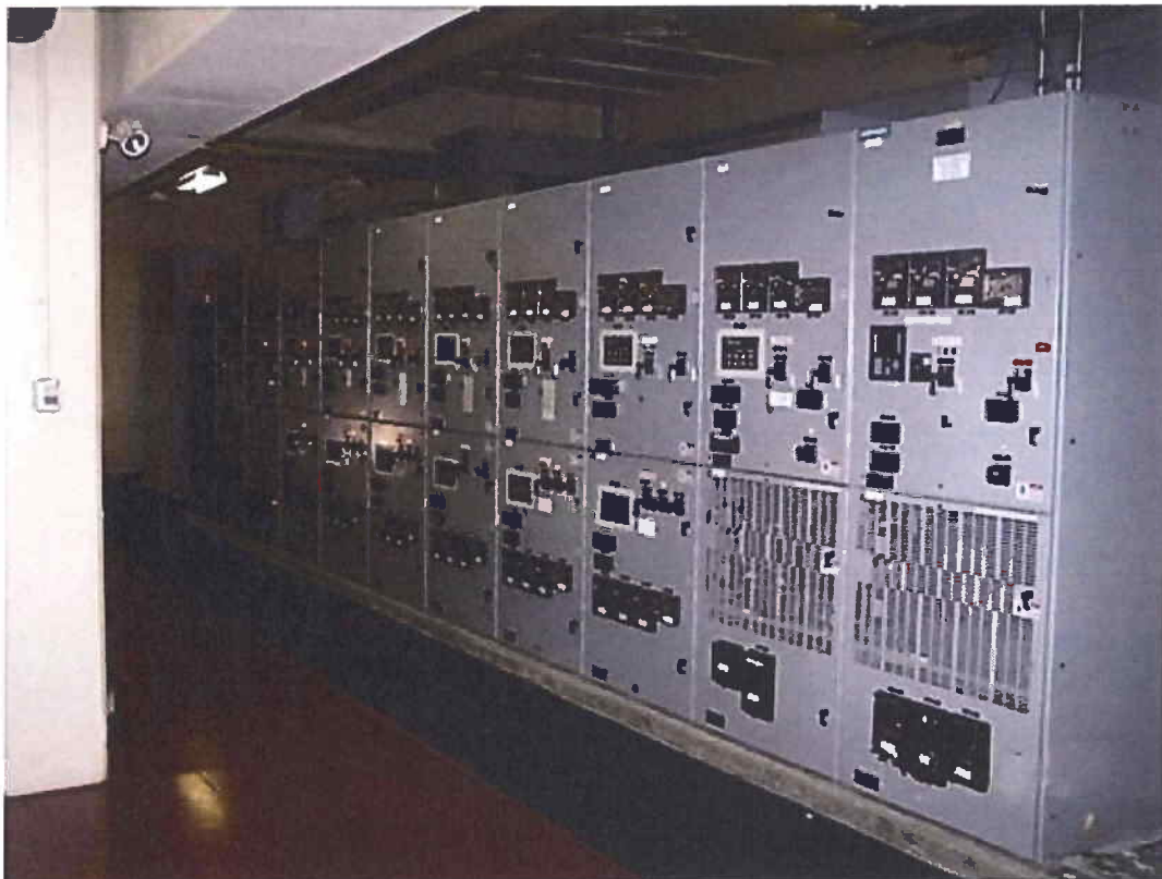
Main Switchgear Building – Medium Voltage Switchgear
