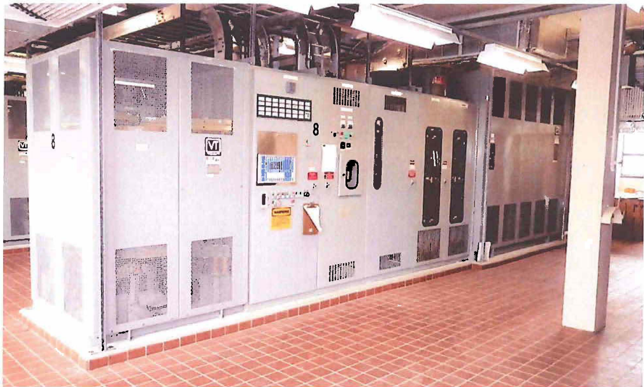
North Main Pump Station VFD for Motor 8 (One of Ten)
