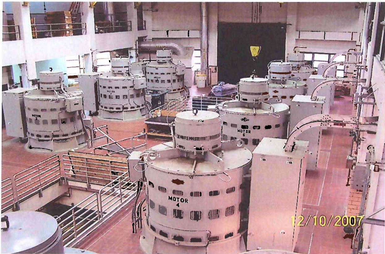
North Main Pump Station Motors/Ten in Total/Pumps are in Lower Level
