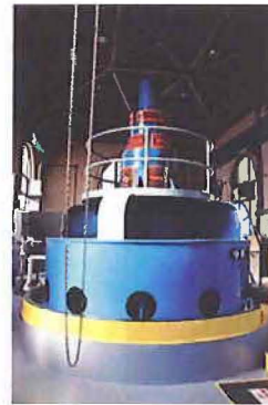
Hydro Turbine at Oakdale
