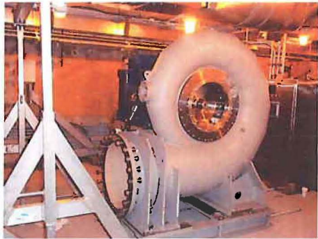
Hydro Turbine at Loring Road
