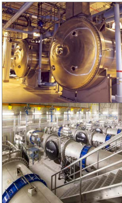
Ozone And UV Generators at the John J. Carroll Water Treatment Plant
