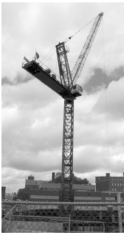
The tower crane at the Union Park DTF site stands 112 feet to the cab. It can handle up to 30,000 pounds of load.
