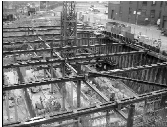
A view of the excavation from the roof of the Pump Station.
