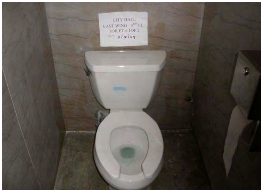
Figure 3.2 Sample Low-Flow Toilet After Retrofit in a Public Building
