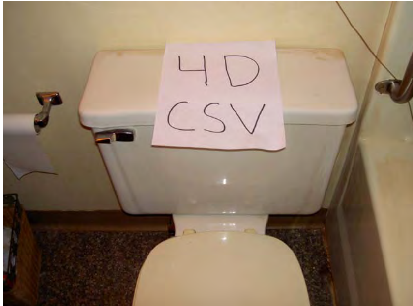
Figure 3.3 Sample High-Flow Toilet Before Retrofit in a Public Housing Unit
